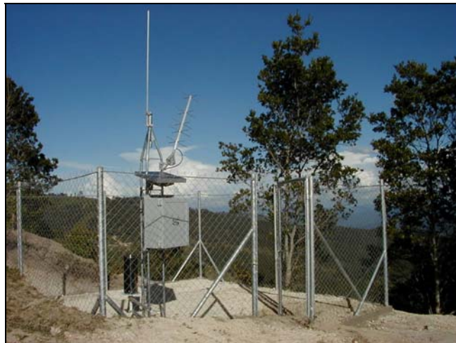
Automatic Rain Gage at Zuzular
