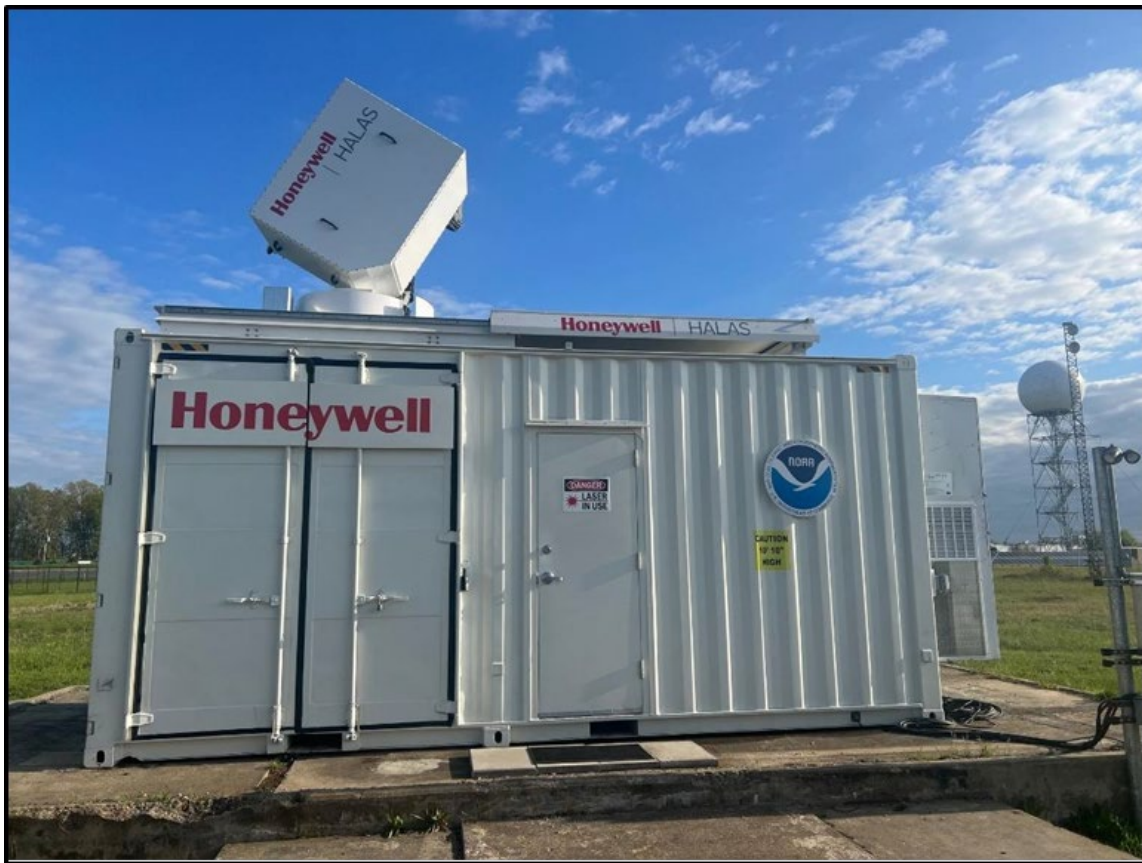
Figure 8: HALAS ground system picture at Sterling Support Center in Virginia.
