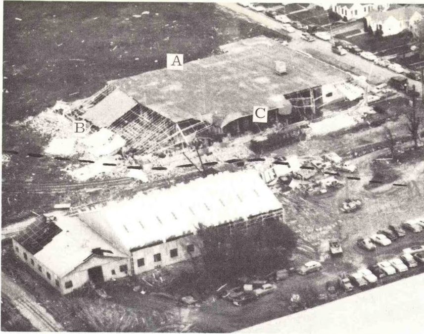
FIGURE 3.—Damage to a building of solid masonry wall construction. Labels A, B, C, refer to walls discussed in text. Dashed line shows approximate path of tornado, moving toward the left.
