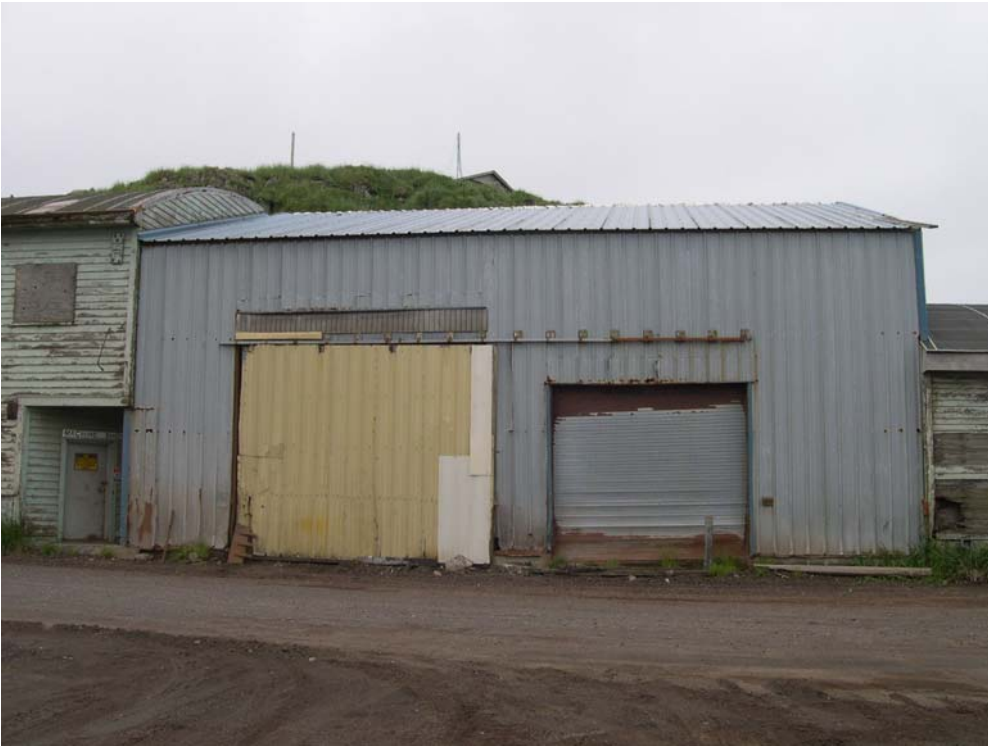
Figure 4. The eastern (front) side of the Connector Building before incurring major damage, July 2004
