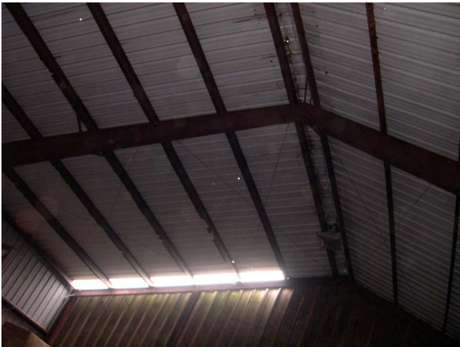
Figure 7. Corroded purlins (near the crack in the roof) and missing roof sheets, July 2004
