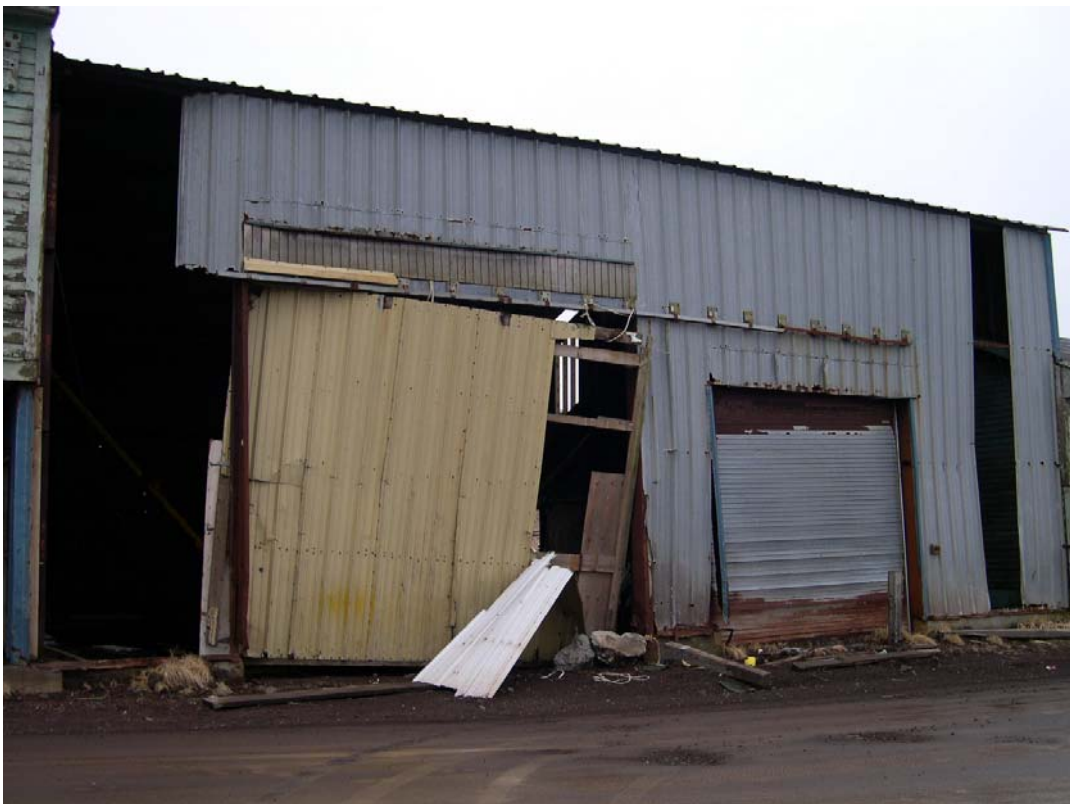
Figure 9. Damaged sliding door and east wall, January 2005
