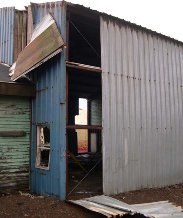
Figure 10. Damaged north and west walls, January 2005
