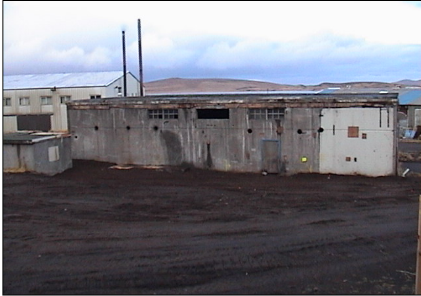
Figure 10. Decommissioned Power Plant site restored to grade at the end of Phase II
