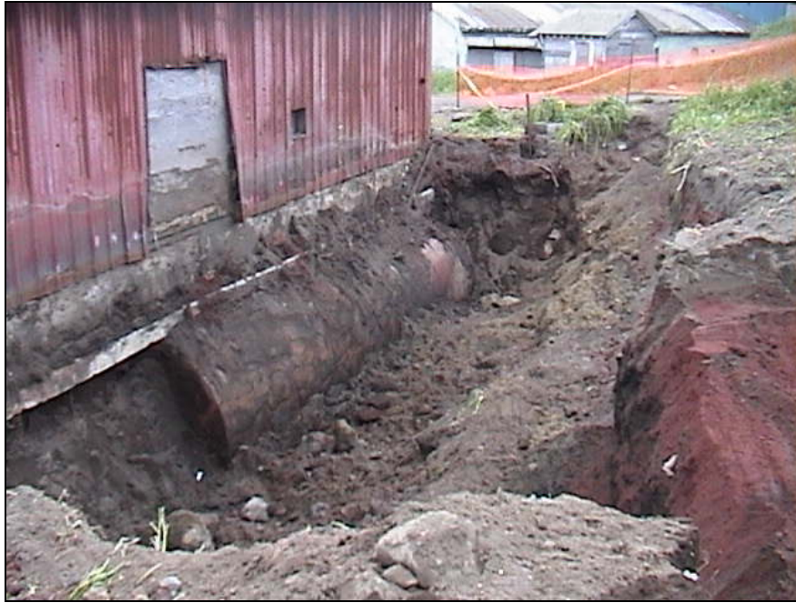
Figure 6. Underground storage tank beneath the Decommissioned Power Plant
