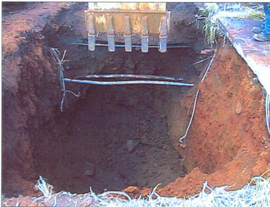
Figure 5. Utility lines and petroleum-stained soil in the UST excavation
