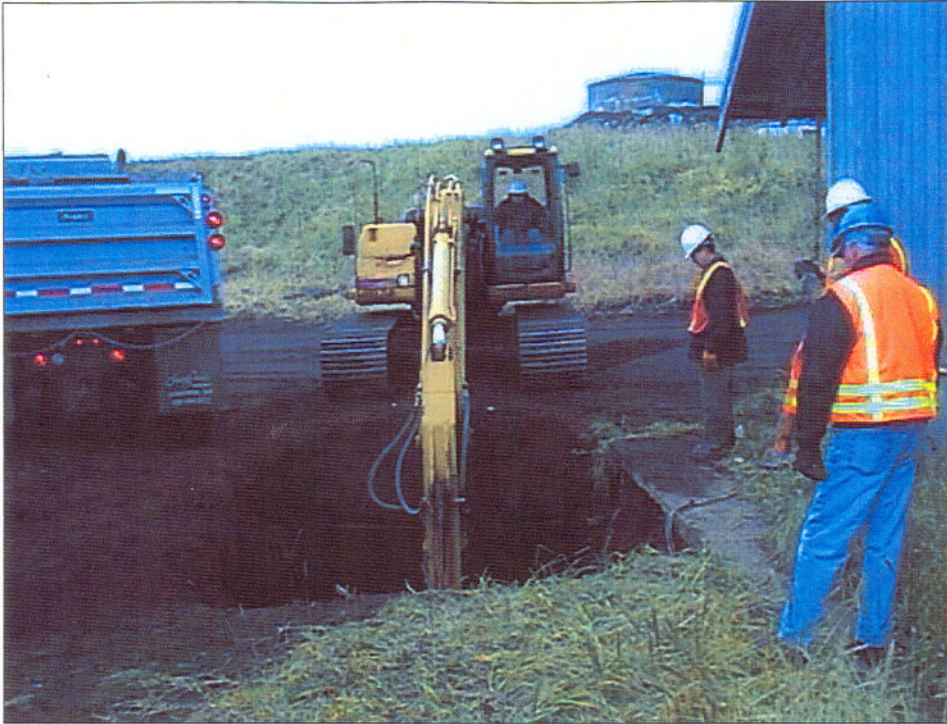
Figure 6. Excavation of petroleum-contaminated soil with a maximum depth of 16 feet below grade
