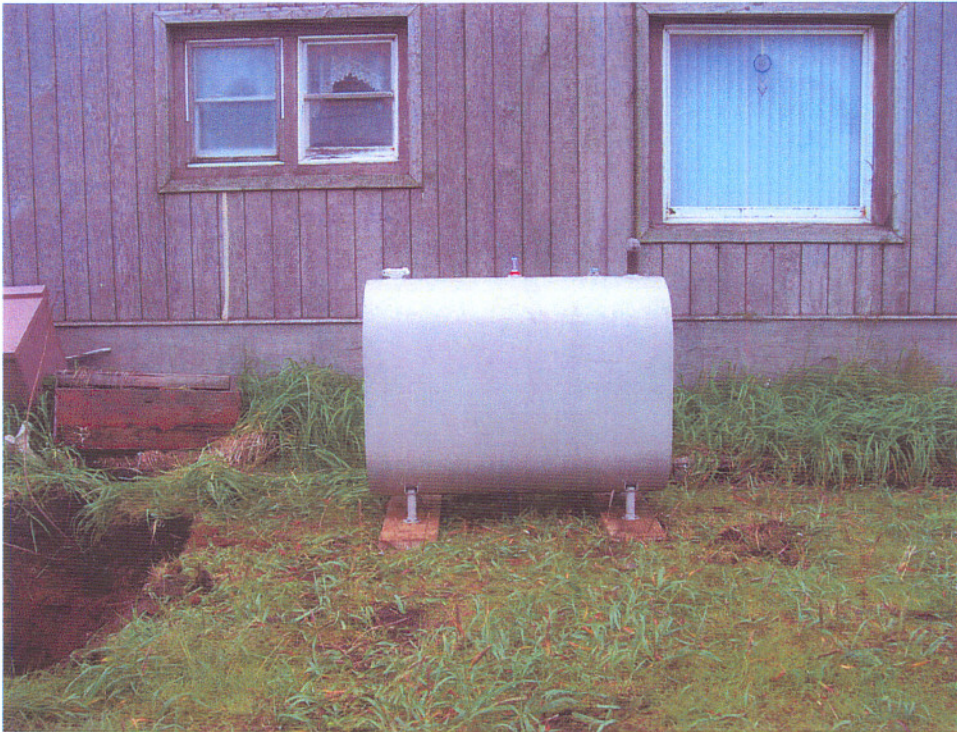
Figure 6. The new aboveground storage tank installed to replace the removed underground storage tank.
