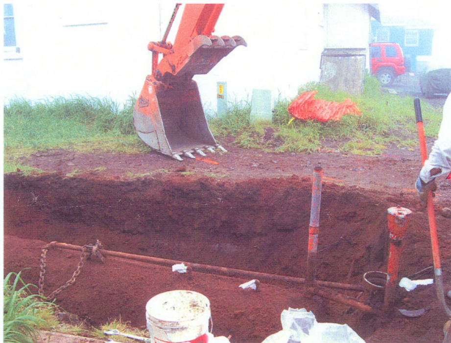
Figure 4. Excavation at the House 102 underground storage tank site. An unidentified cement utility line discovered at approximately 3 feet below ground surface can be seen along the boundary of the excavation.
