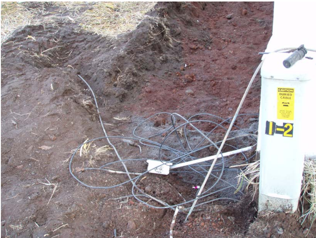
Photo 10. NTPA Site 60. Buried Telephone Lines, NW Corner,TH101. NOAA. 10/2006
