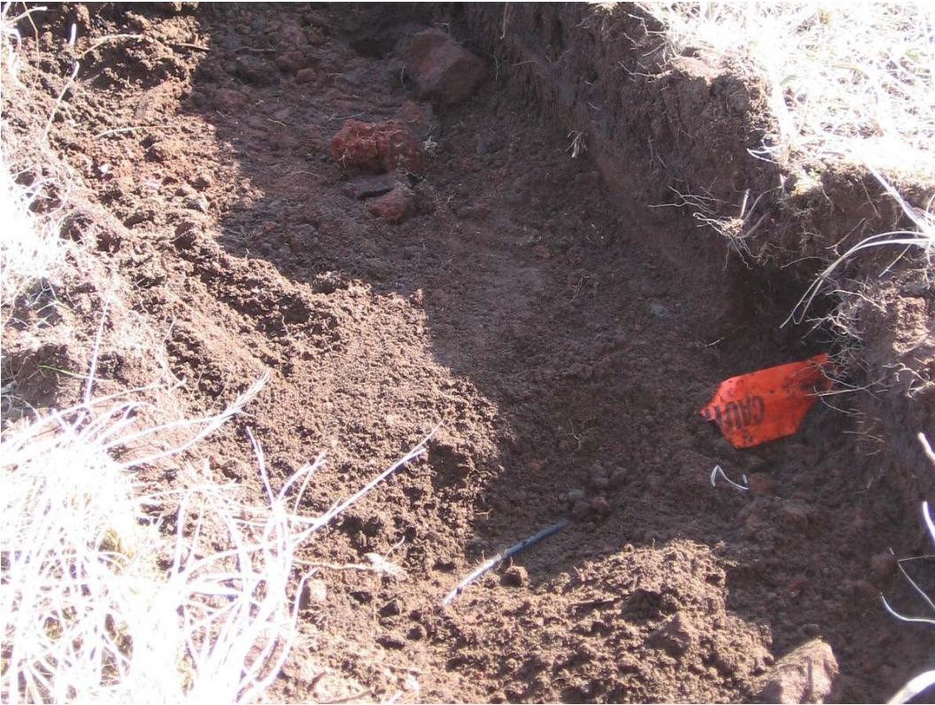
Photo 4. NTPA Site 60. Buried Cable TV Wire, NE Corner, TH101. NOAA. 6/2006.
