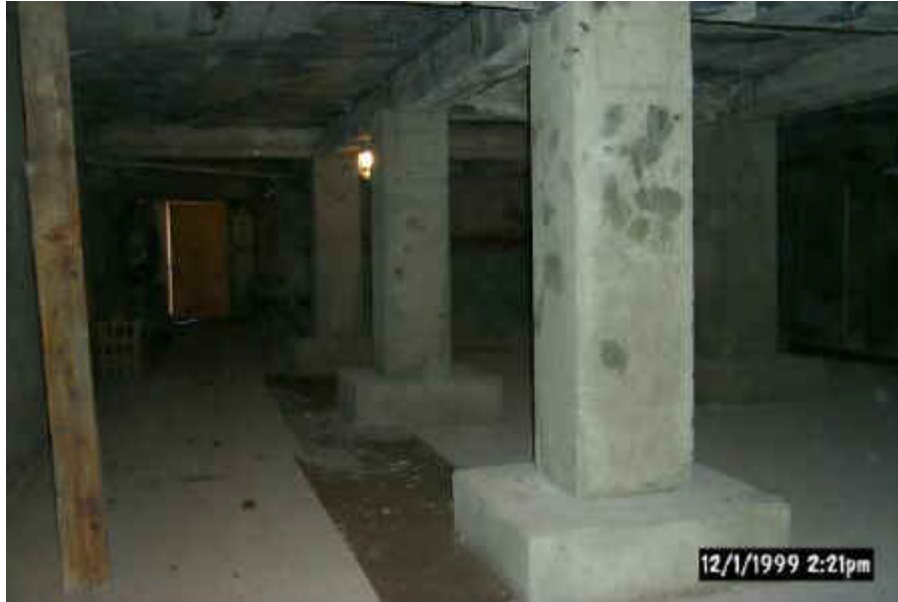
Figure 9. Oversized Interior Columns in the Blubber House Basement
