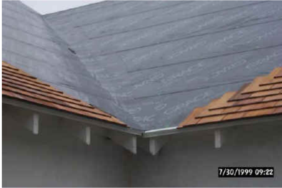
New roof installation. Note the use of ice and water shield over the entire roof area.
