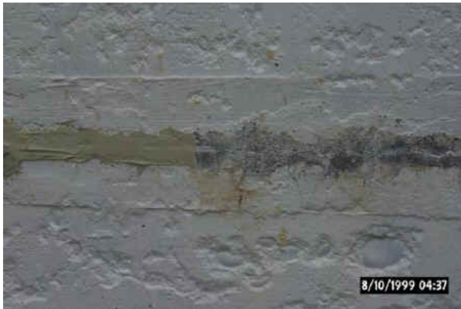
Figure 11. Repaired Crack with Capping Paste Still Covering the Left Side
