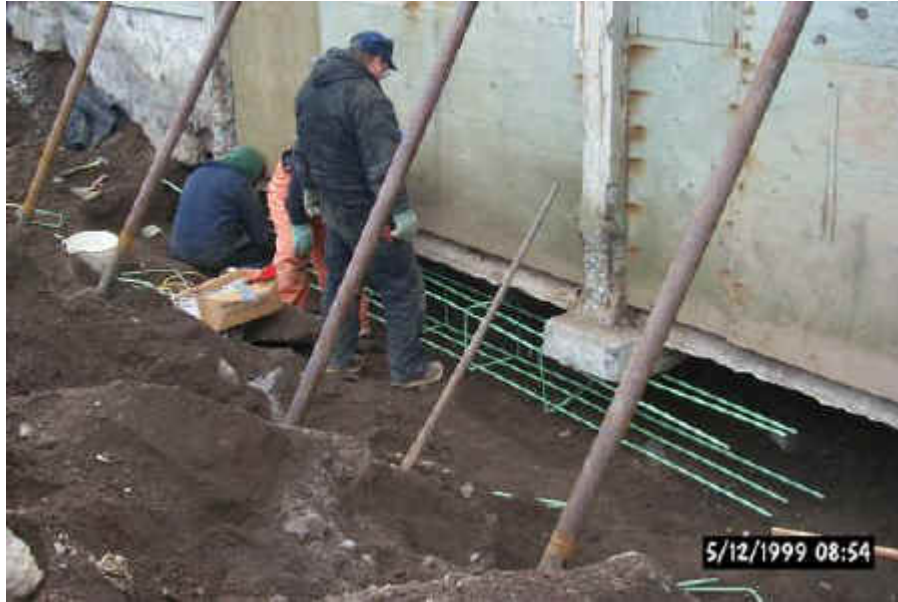
Installing grade beam rebar under the existing slab and exterior columns of the blubber house basement.
