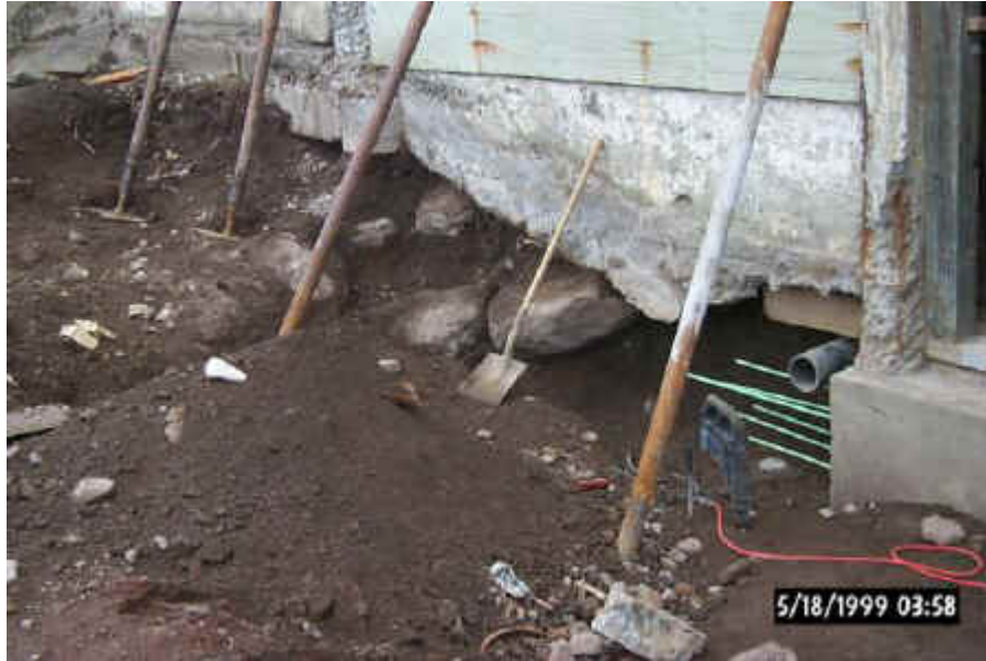
Figure 8. Large Rock in Path of Perimeter Grade Beam Construction
